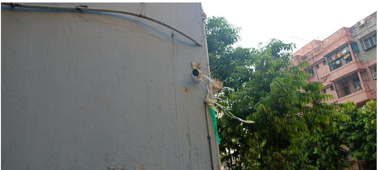
CCTV Cameras in various areas
